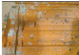
Clay tile from the home of Tony Rupcic's mother in Senj, Croatia built in 1902; that roof is still in good condition. There are many intact 120+ year old clay and slate roofs throughout Europe. Just Google "Senj Croatia" to see for yourself!
